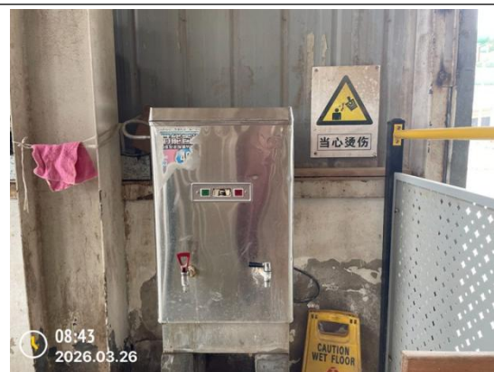
Drinking water device
