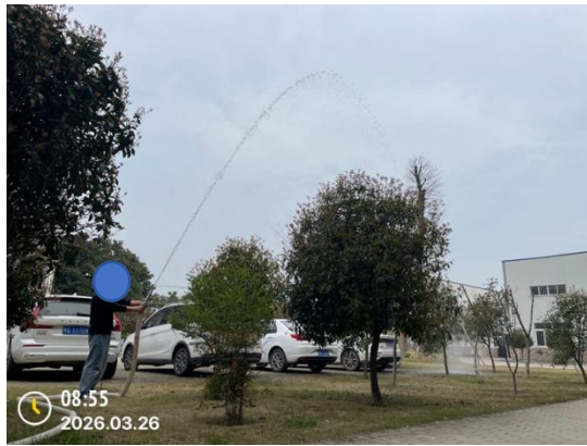
Fire hydrant testing
