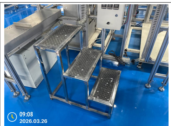
NC-7.17 Two ladders at workshop were missing handrail.
