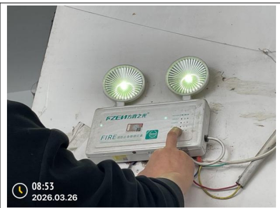
Emergency light testing
