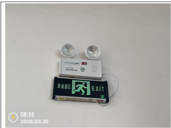
Exit sign and emergency light
