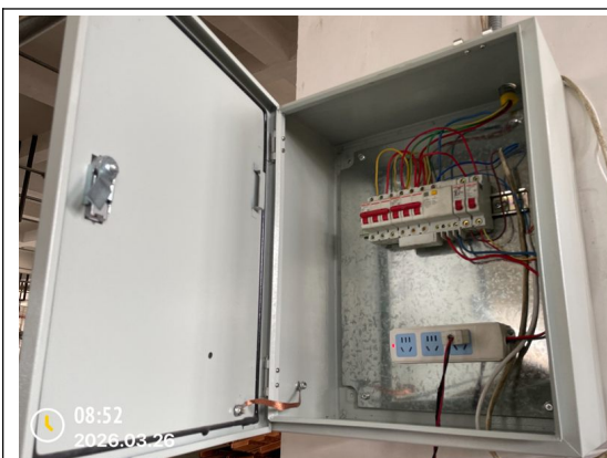
NC-7.13 One sampled electrical switch box was found without inner cover and outer cover was not closed.
