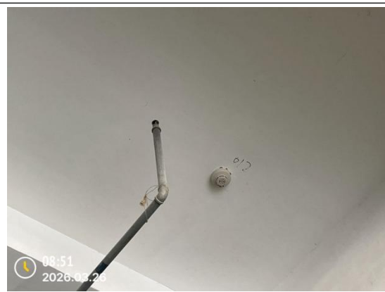
Smoke detector and sprinkler
